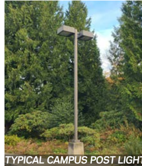
TYPICAL CAMPUS POST LIGHT
