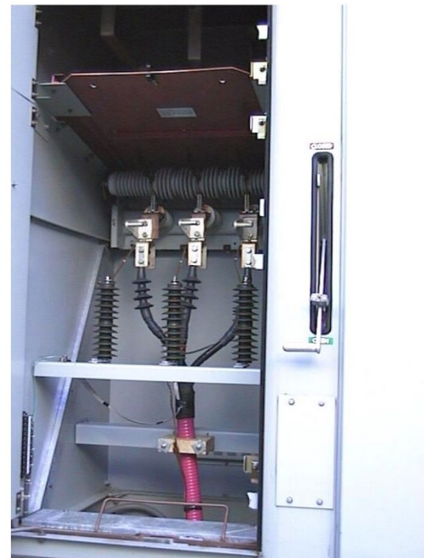
16K – Figure 4 Barrier Isolating Switch
