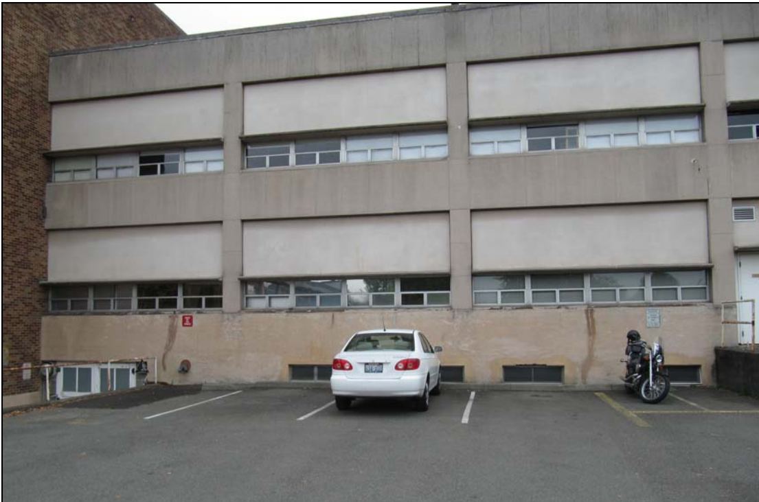
Figure 17. Below, detail view of a portion of the south façade showing deteriorated stucco cladding and non-original, solid infill above the remaining windows.
