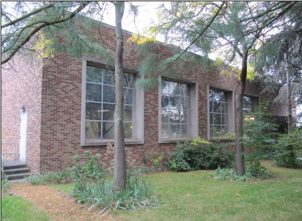
Figure 15. Below, view looking southeast at a portion of the building's northwest corner. The proposed project will involve removal and replacement of the large windows shown in the west facade.
