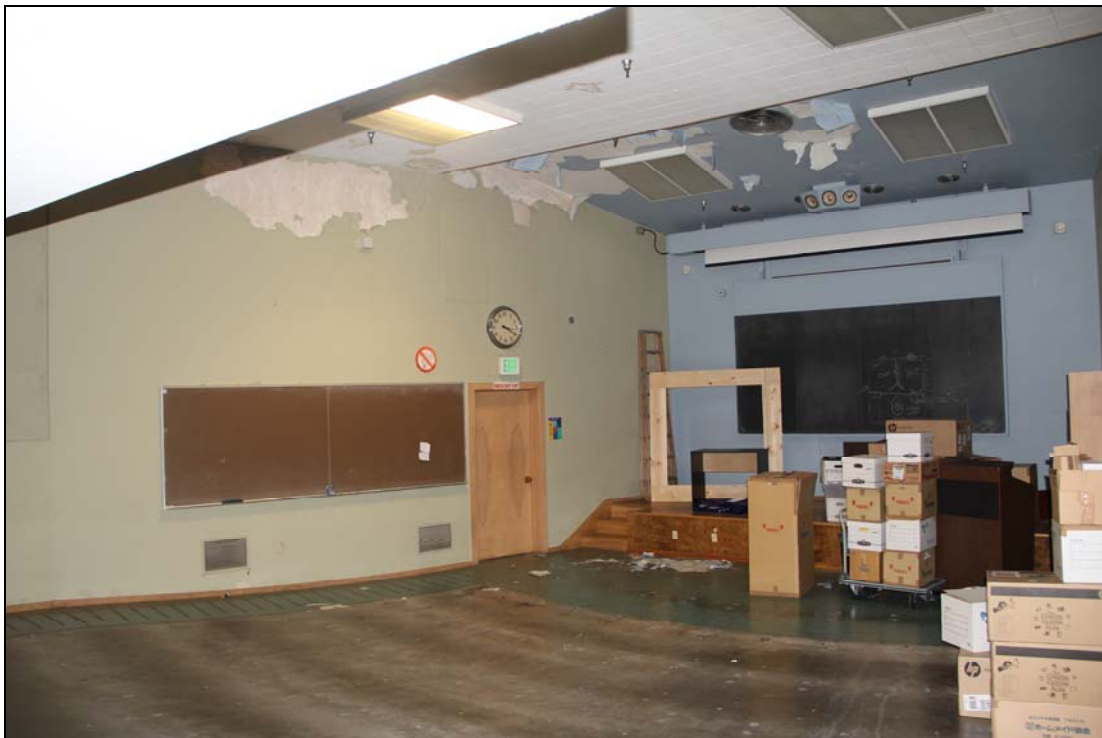
Figure 26. Below, interior of the existing auditorium space in the former Fisheries Center.
