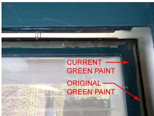
Window Detail showing multiple layers of green paint
