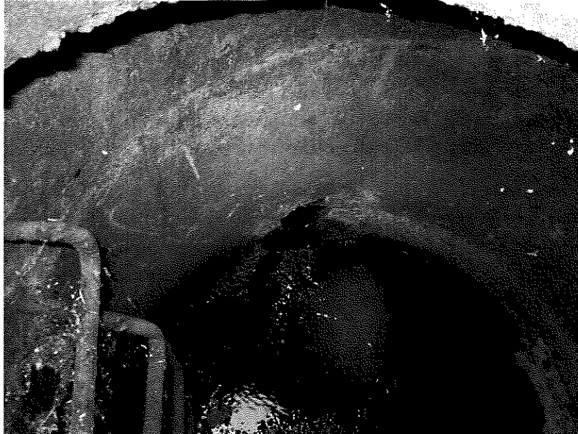
Figure 14 Overflow 2 – 6 Inch Pipe
