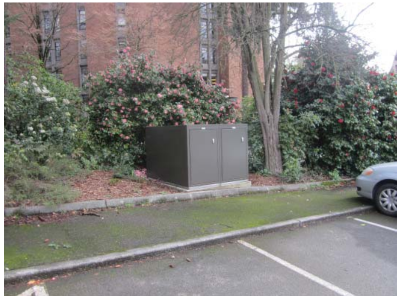
Existing bike locker at Communications Building - using a University Standard "dark bronze" color.
