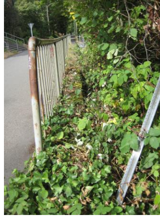
Looking north, detail along eastern edge of bridge, with non-original metal railing 2013
